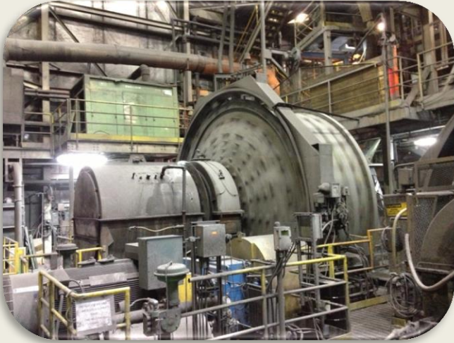
Greens Creek mill facility
