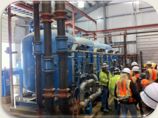
LMPT touring Kensington Water Treatment Facility
