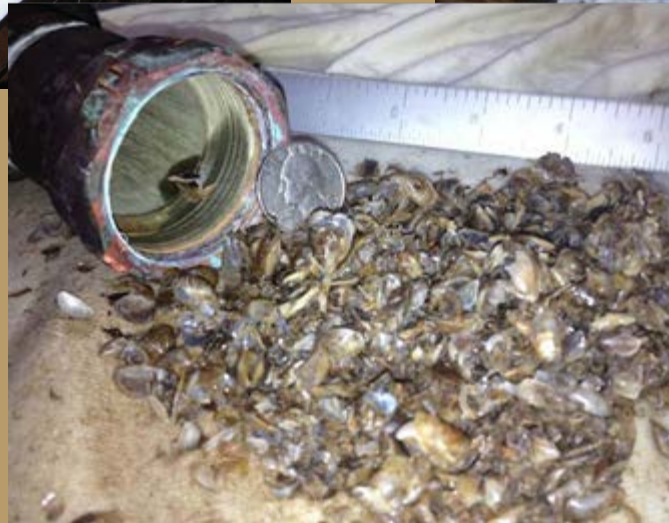
Shell debris from thrust bearing cooler piping
