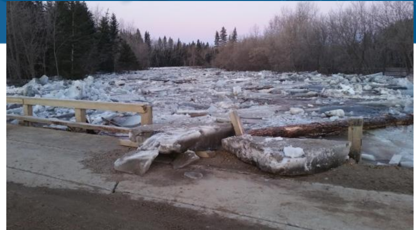
Ice jam damage to bridge, Torch River, Manitoba 2017 - Regional Municipality of Torch River
