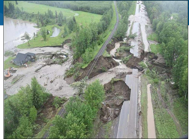
Washout of Highway and Railway, Peace River Country, B.C. 2016
