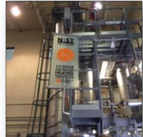
One-third scale NIST-1 Test Facility
