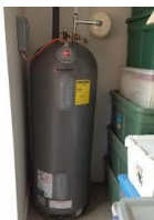
Electric Water Heaters: (.4 - .7 kW)
